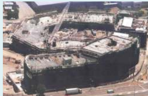
Sydney Park housing complex with 922 apartments. This eight storey building is without RCC columns and beams. The entire structure is built on Gypcrete® /Rapid wall panel.
